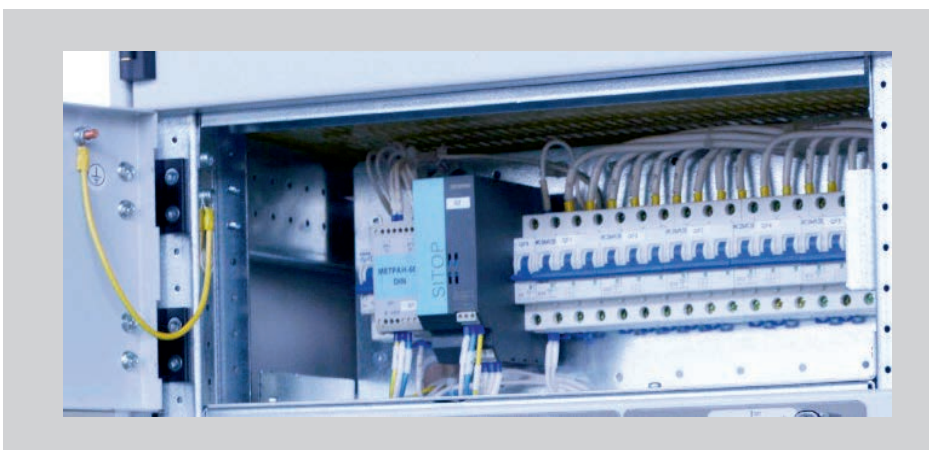
Stationary cabinet cell
