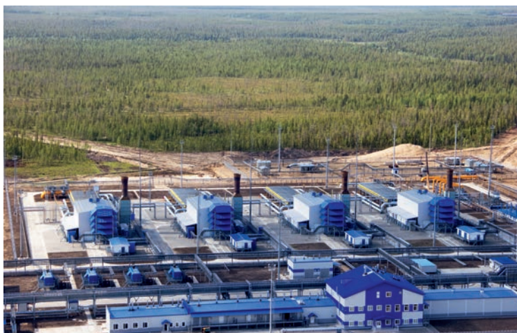
GPA-32 "Ladoga" at CS-8 "Chikshinskaya", "Bovanenkovo-Ukhta" gas trunk line
