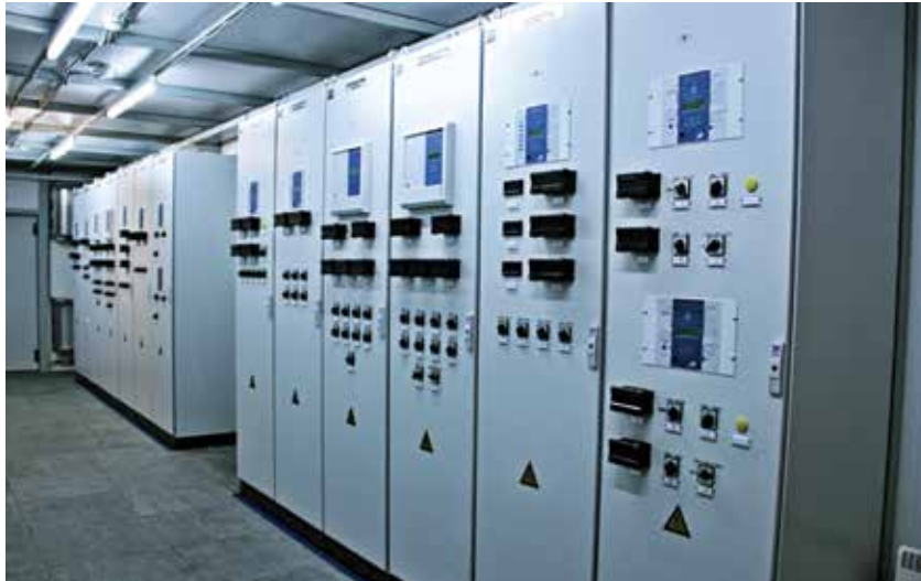
Cabinets of power protection and automatics in a container unit
