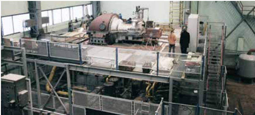
Steam turbine test bench
