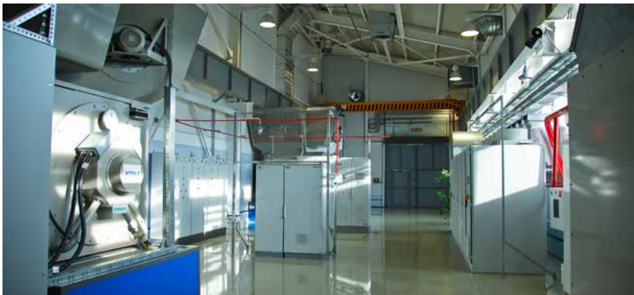
4.0 MW EGPU at CS "Volodino" of the Main Gas Transfer Pipeline "Parabel-Kuzbass"
