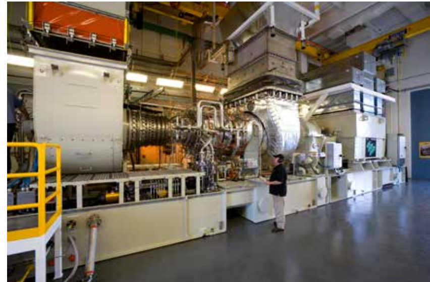
GTU-T25 on the test bed
