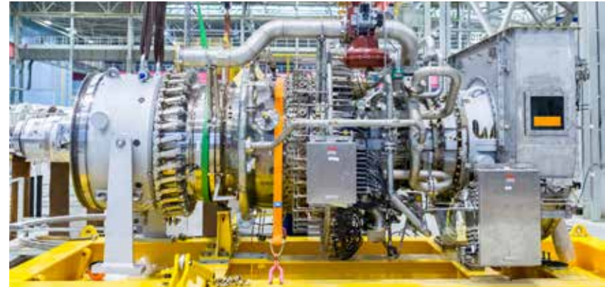
Gas turbine unit T16
