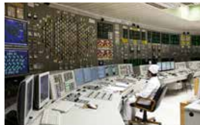
Modular Control Board of the 2nd power unit of Kurskaya NPP
