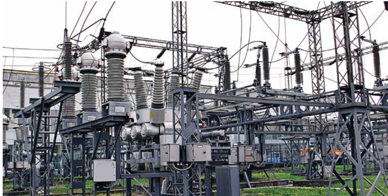
Outdoor switchgear-ОРУ 110 kV
