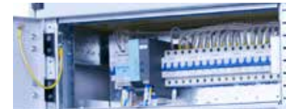
Stationary cabinet cell
