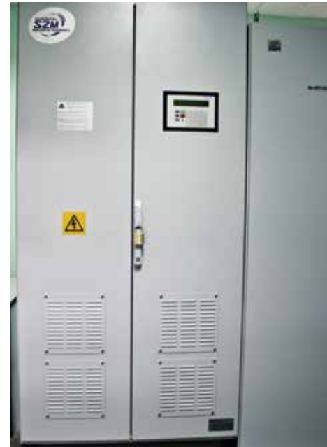
Active magnetic bearing control cabinet
