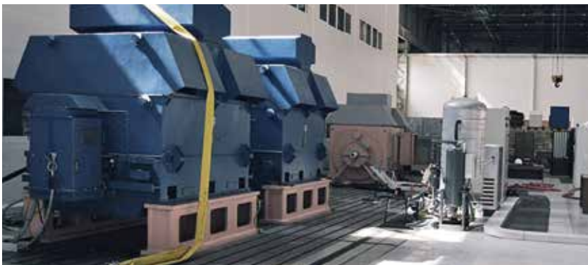
Electric drive test bench
