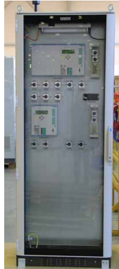
Protection Relay and Control Cabinets
