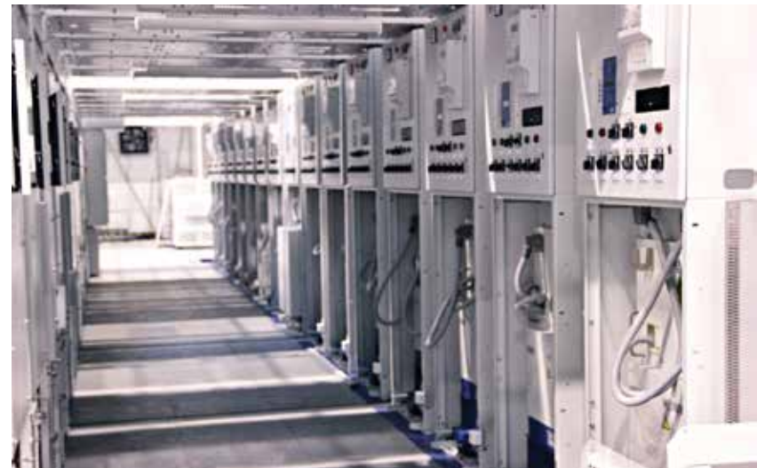
Factory-assembled switchgear in a container unit
