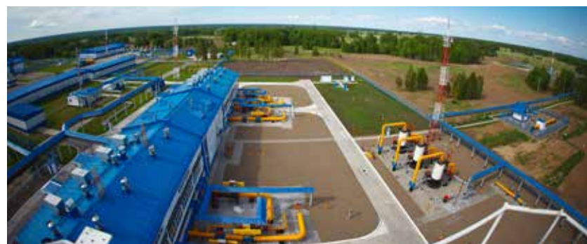
EGPA 4.0 MW on CS "Volodino" of the main gas transfer pipeline "Parabel-Kuzbass"
