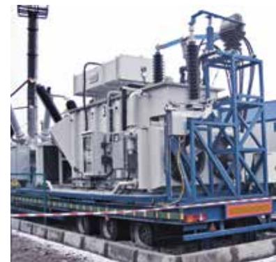
JSC Lenenergo Substation № 124
