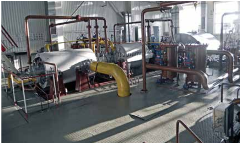
K320-131-1 centrifugal compressor at the Severo-Danilovskoye field TPP compressor station
