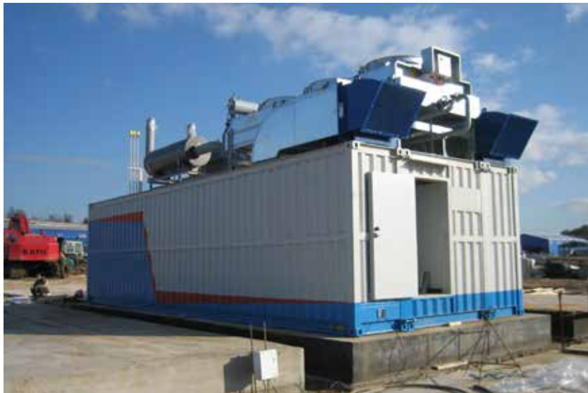
Gas-Piston Power Plant on CS "Kazachya"
