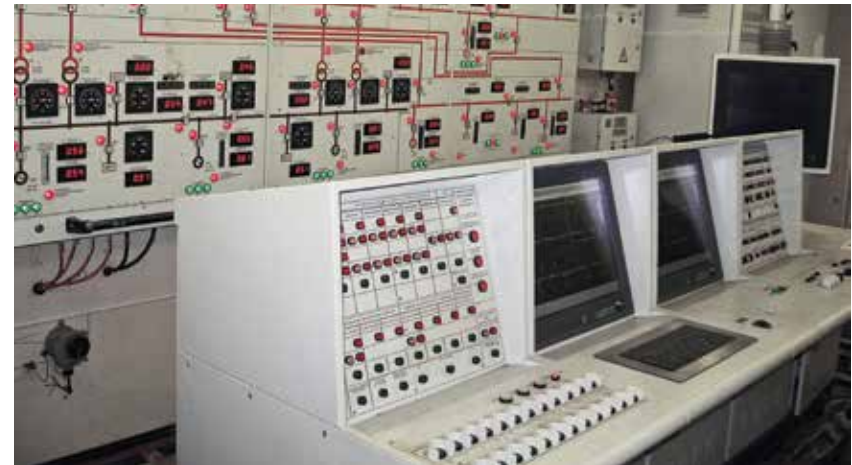
Integrated Control System of the Vessel Technical Equipment
