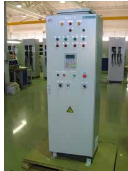
The control cabinets (ЩО-3, ЩД-3)
